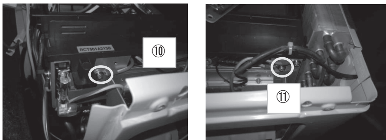
Fig.5 Earth cable of control box
