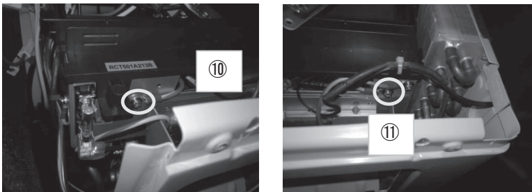
Fig.5 Earth cable of control box
