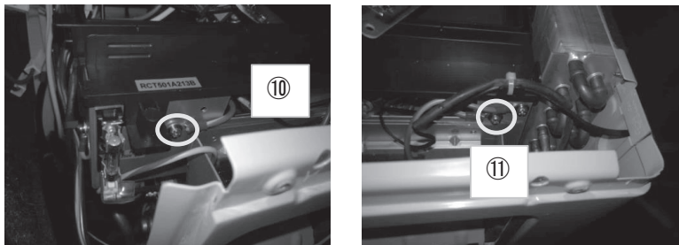
Fig.5 Earth cable of control box
